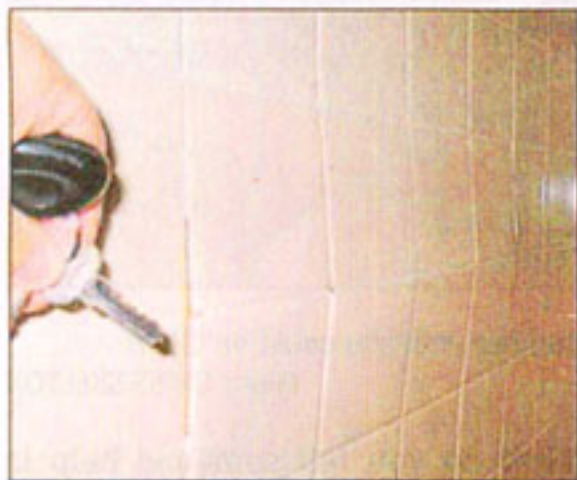
Andrew was right: The tiles really were coming off the walls in the bathroom.
